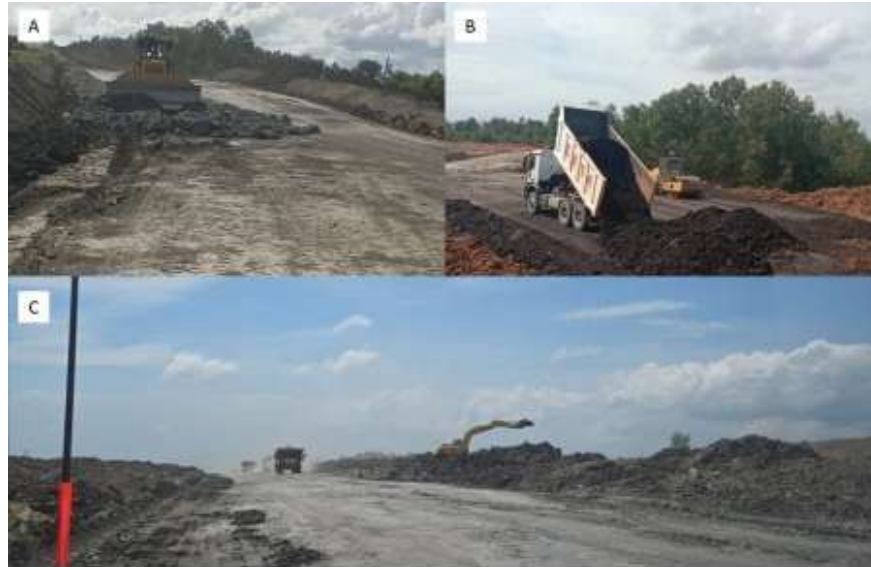
Figure 2. Hauling road resurfacing using claystone material at (A) Persiraja Road; (B) Semen Padang Road; (C) Road Condition after Layering.
